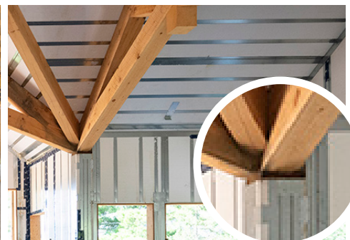
When a close-up photo is warranted (ie. a beam pocket) take a photo further back first, then close up.
