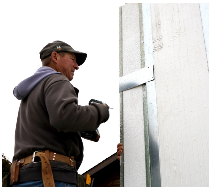
Plumb both ways and secure with the outside corner connector. Screw to the bottom track so the panels cannot move.
