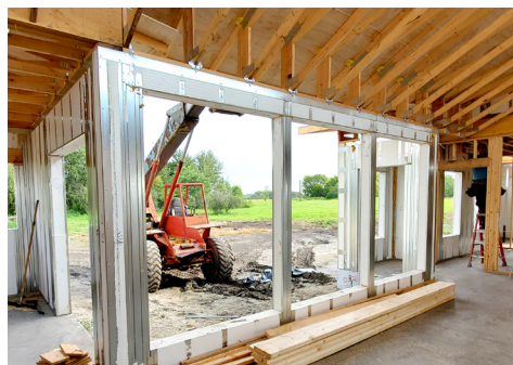
Take Interior photos from as far back from the wall as possible, and include 15-20 foot sections of wall per photo.
