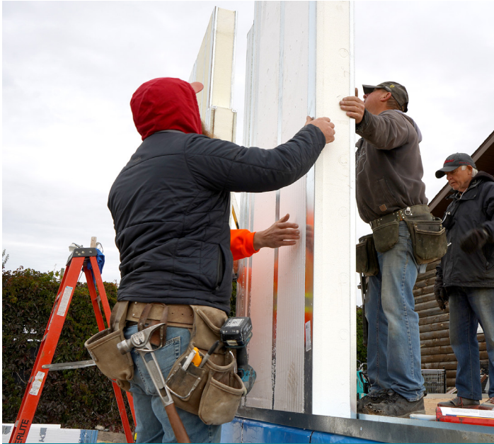
Opening size & placement must be as per installation drawings. Adjust panel placement at openings accordingly as per layout.
